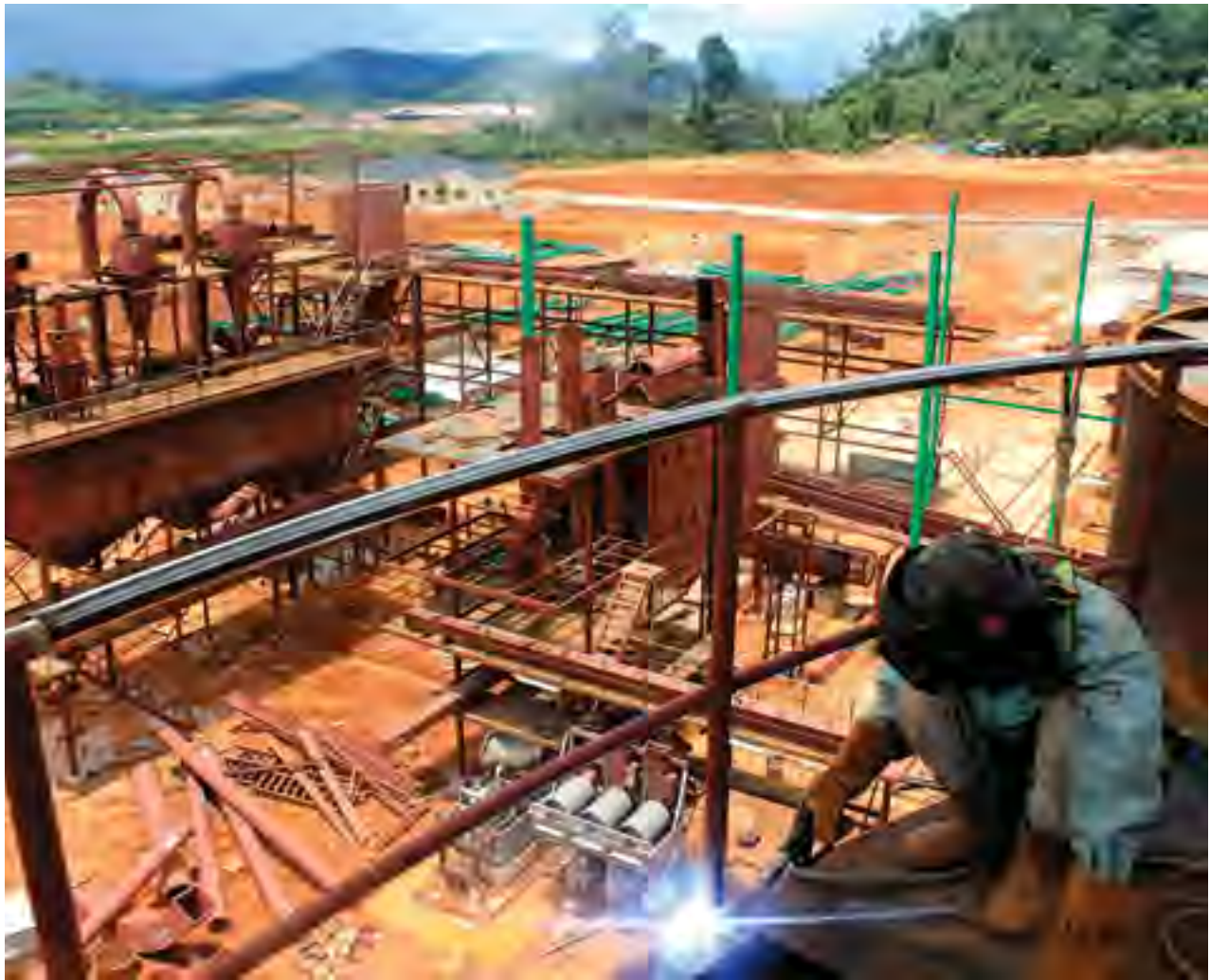
Progress on the full-scale mill at our West Kalimantan Plantation in 2015. It is due to be finished by the end of 2016.
