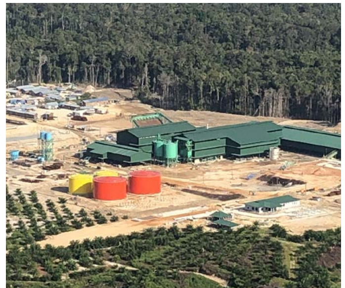
Construction Progress of New CPO and PKO Mills at West Papua Photo: Corporate Communications
