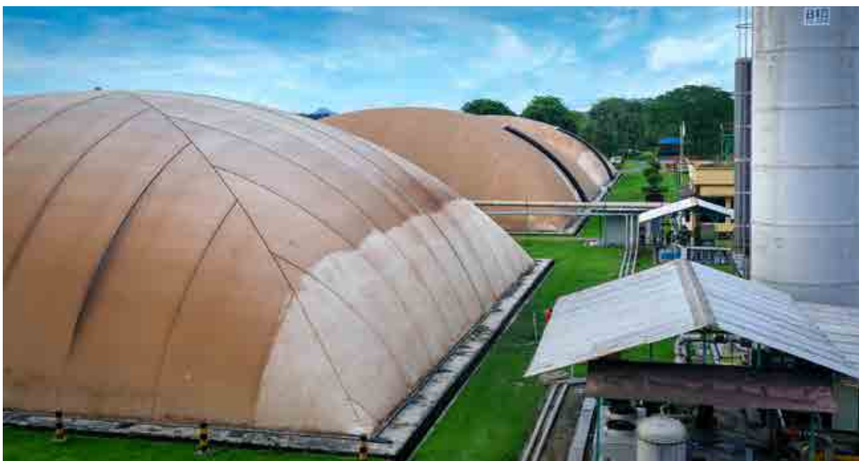
Our Biogas Plant in AANE, East Belitung
